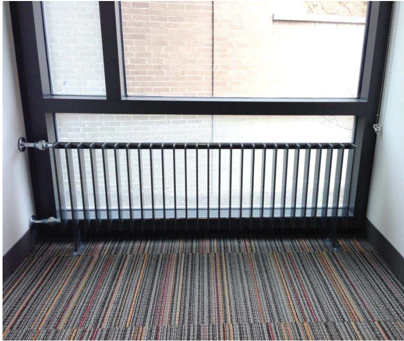
Maximize Daylighting: Panel Radiators at Perimeter with Frit Glass Lower Window Section
